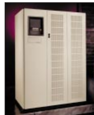
The Powerware 9315 is capable of powering the entire operation for 38 minutes. But Interpath went one step further and installed a 1750-kilowatt diesel generator to feed the UPS in the event of a power outage. The generator kicks in just 7 seconds after detection of failure of the incoming power. Even if the generator is used, the UPS continues to condition the power. Unconditioned generator power is often "dirty" and can cause problems with the operation of sensitive equipment.
